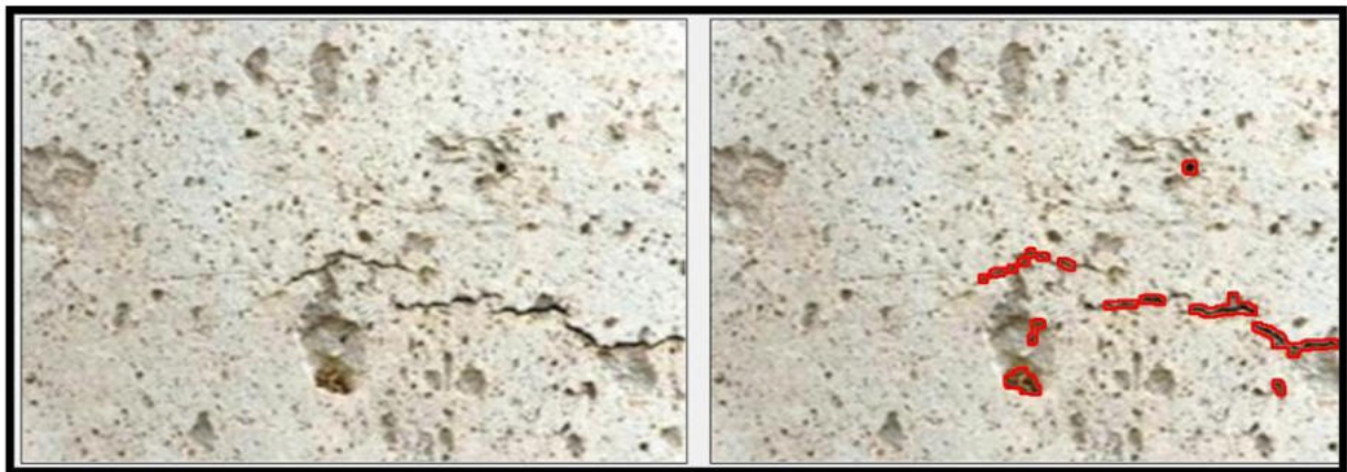
Picture 20: Detected segmented cracks
